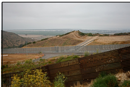
Triple wall construction on the U.S. side of the San Diego/Tijuana, Mexico border.
